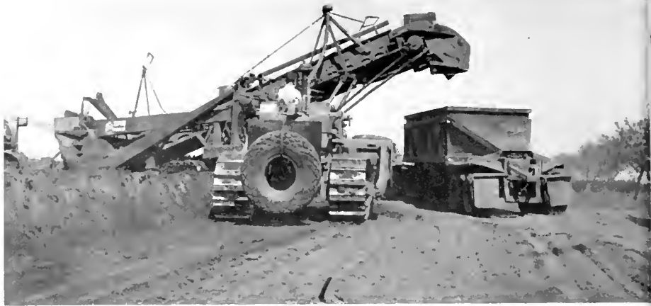
Crawler-type belt loader pulled by a tractor required push equipment in deeper cuts
